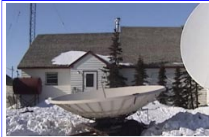
The old satellite dish rests on a trailer in the snow. The tower to be replaced can be seen standing behind the building on the left.
